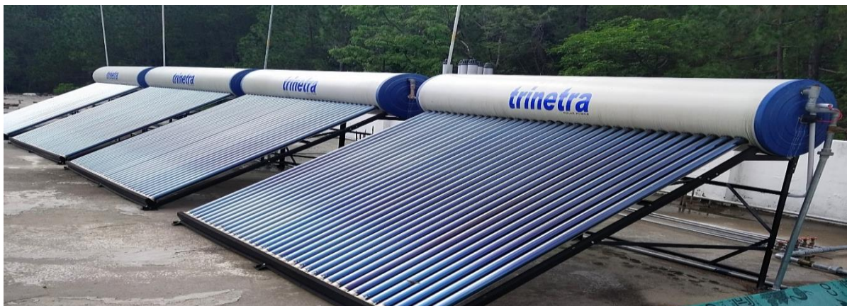
Solar thermal panels for hot water supply of the campus
