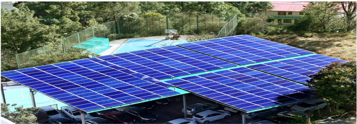
400kWp grid-connected Solar Photovoltaic Power Plant at Shoolini University
