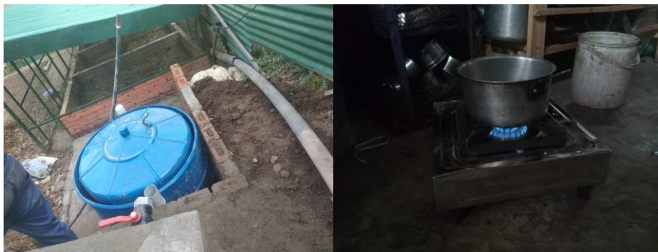
Figure 12: Biogas system installed in agricultural farm at Shoolini University
