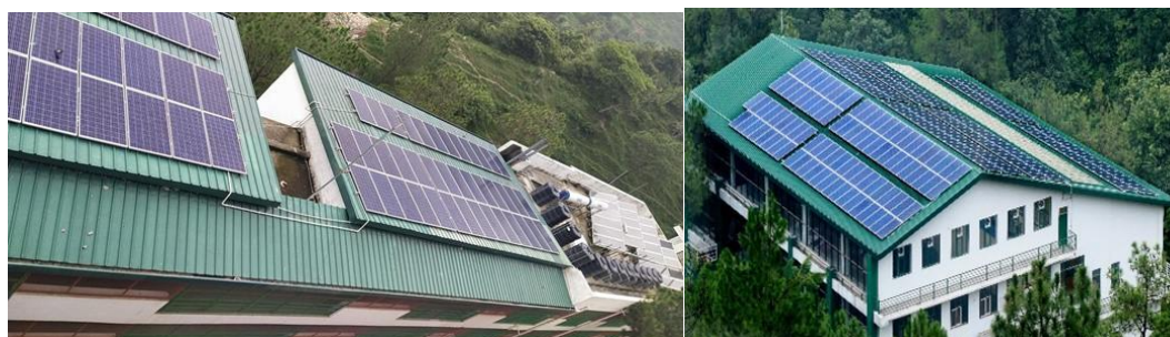
Figure 1: 400 kWp PV power plant installed in the university
