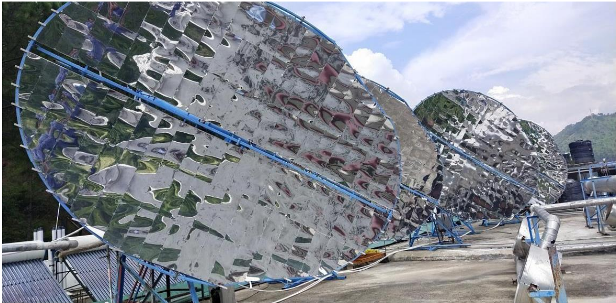
Figure 11: Steam cooking system for 500 students at Girls' hostel rooftop at Shoolini University
