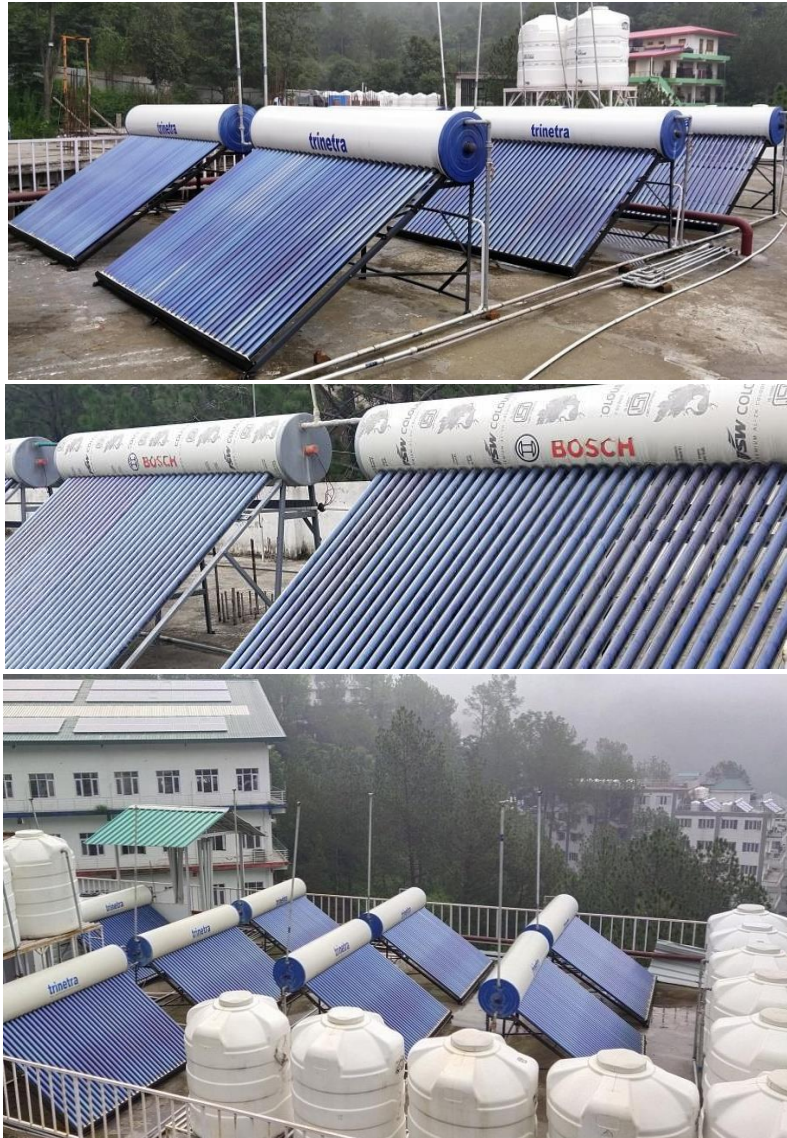
Figure 5: Installation of 38000 litres per day solar water heating systems in the university campus.
