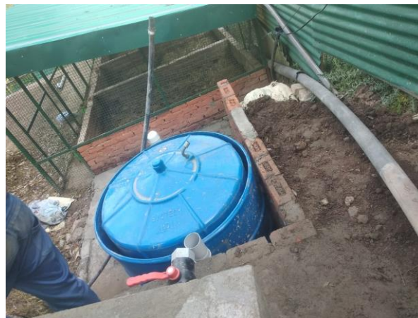
Figure 7: Biogas plant for cooking installed in agriculture farm in Shoolini university
