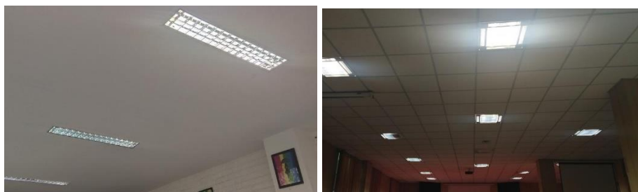
Figure 11: 20W LED lights installed in the University
