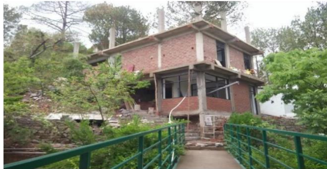
Figure 18: Animal House building at Shoolini university being built with integrated Trombe Wall for better energy efficiency and thermal comfort
