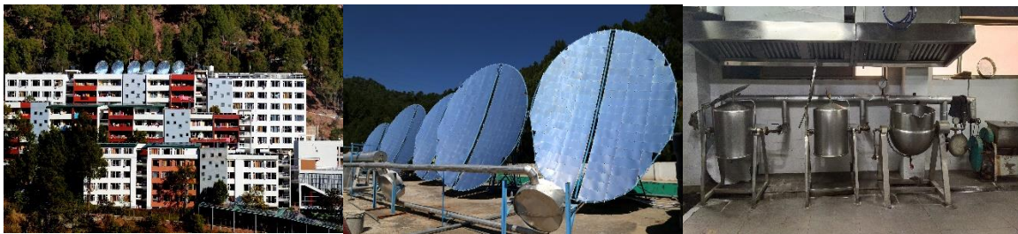
Figure 4: Concentrated solar steam cooking system installed on roof top of the girls hostel at Shoolini University
