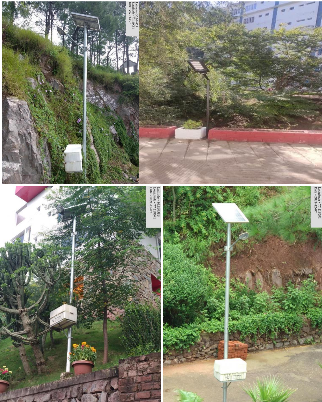
Figure 9: Solar streetlights installed in the University campus.
