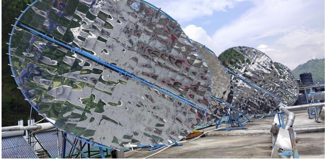
Figure 3: Concentrated solar powered community steam cooking system
