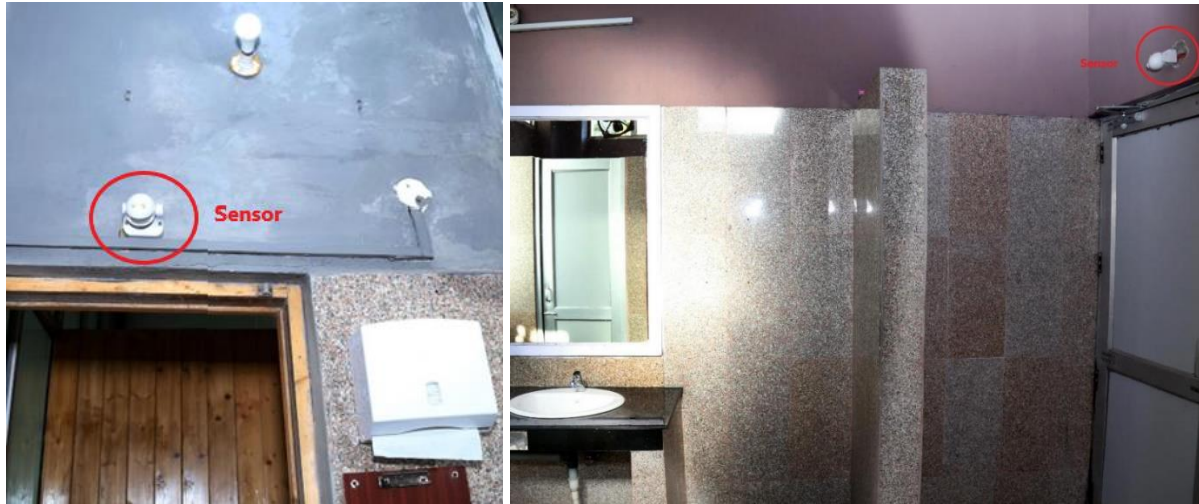
Figure 8: Sensor based lights at various restrooms have been installed. These sensors detect the presence of a person and turn off when there is no human presence in the rooms.
