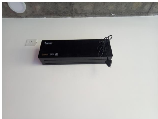
Figure 13: Energy efficient PTC air heaters have been installed all international hostel rooms
