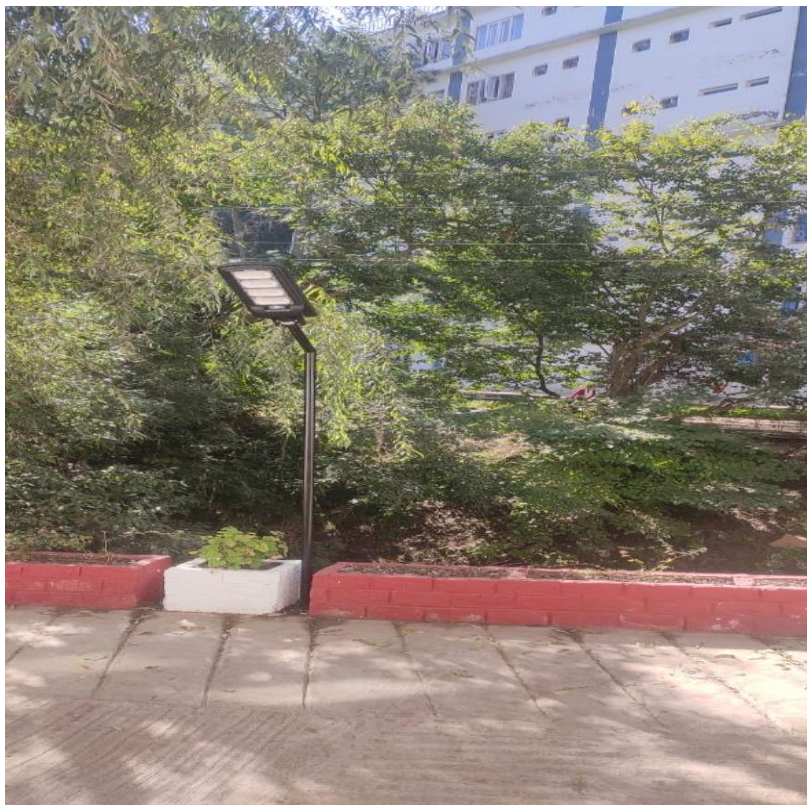
Figure 13: One of the LED street lights within the university campus
