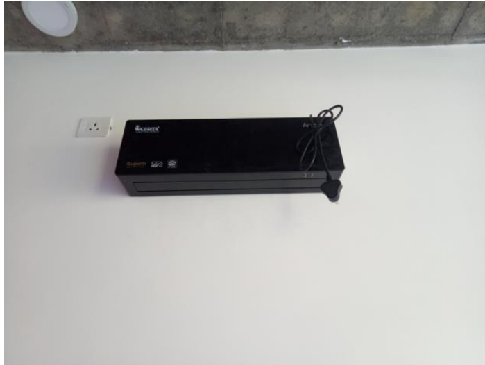
Figure 8: Energy efficient PTC Air heaters have been installed all international hostel rooms
