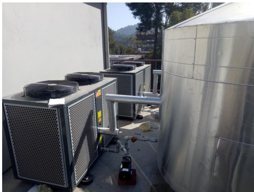
Figure 7:Energy efficient heat-pump based water heating system has been installed in the international hostel Shoolini University
