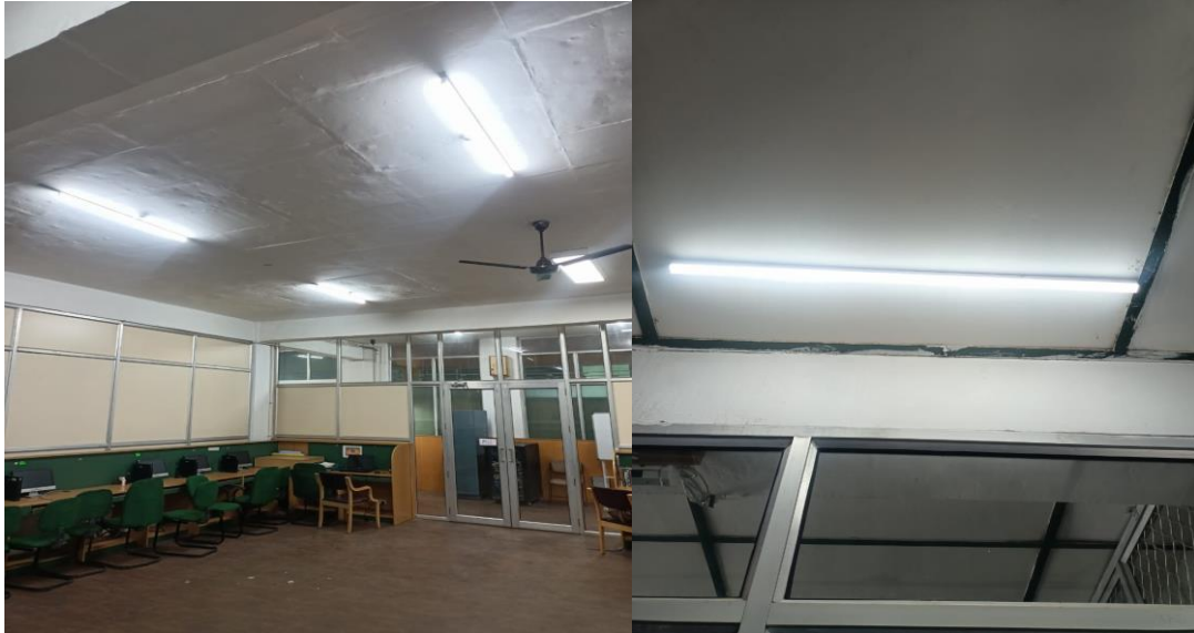
Figure 12: LED lights are being used in almost all buildings in the university
