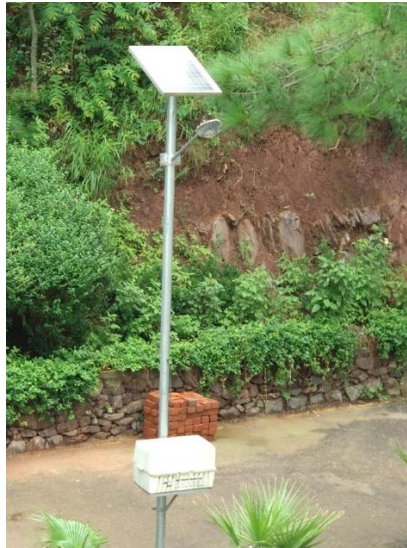
Figure 5: One of solar street lights installed in the campus
