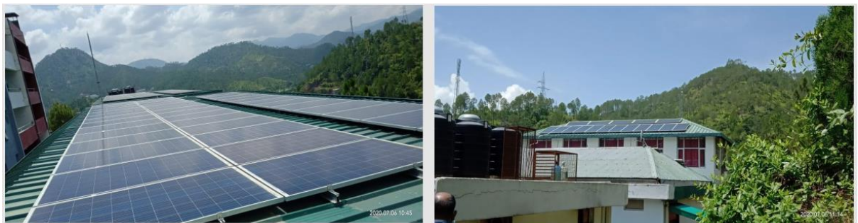
Figure 1: PV Power plant installed on various buildings of Shoolini University
