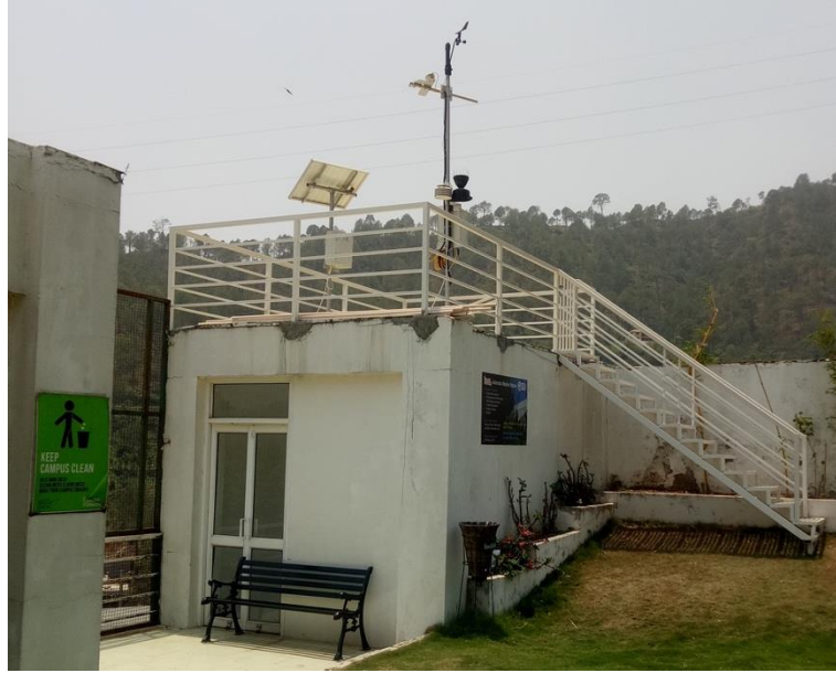
Figure 4: Automatic Weather Station installed on top of Library Building at Shoolini University
