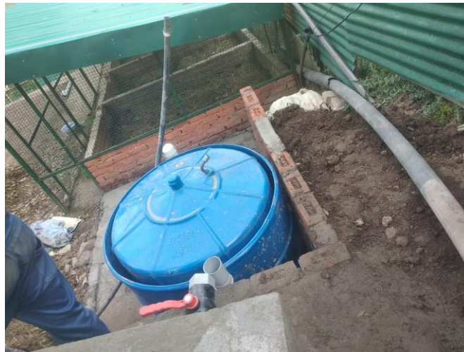
Figure 2: Biogas system installed in Shoolini University
